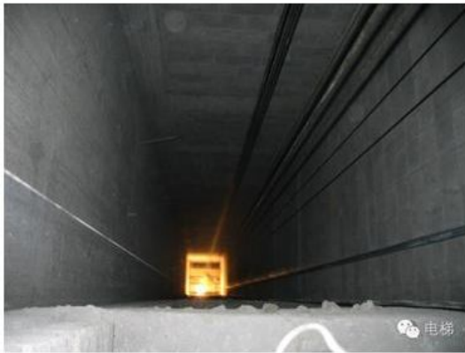
Steel rope and travelling cable appear inside shaft
