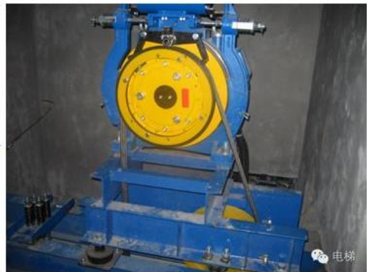
Machine steel rope installed
