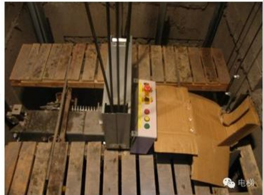
Elevator can run after COP fixed
